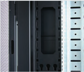
Backside with a pair of vertical cable management
